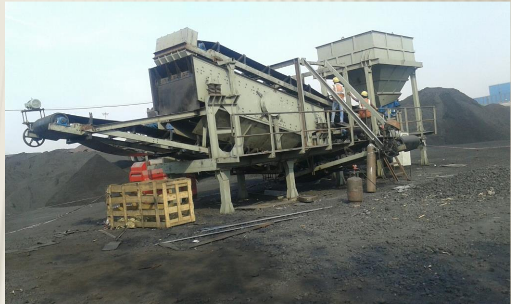
Stationary crushing & Screening Plant at TATA STEEL PLANT
