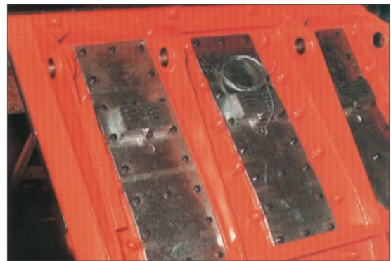
Heating system with electrical heating elements
